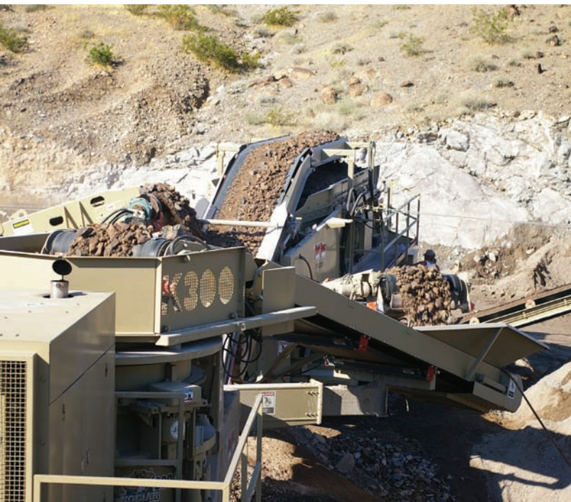
After screening, anything larger than the desired 19mm minus material goes back to this JCI FT300 track-mounted cone crusher.
