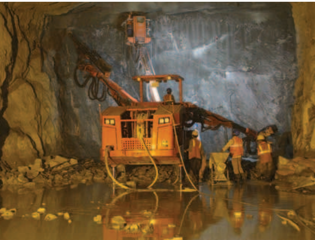
Sandvik has supplied four DT 820 underground drill rigs to Hindustan Construction Company (HCC) for construction of India's first underground crude oil storage cavern, at Vizag. The budget for cavern construction on 1.33 million tonne capacity facility is INR 375 crore (US$ 81 million).
