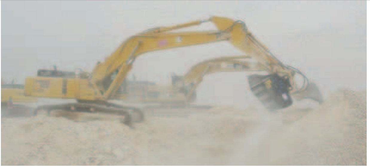
MB Crusher has supplied a BF120.4 crusher bucket to the project to upgrade 600 km of the NH7 between Hyderabad to Bangalore. The unit is being used to produce 40 mm aggregates.
